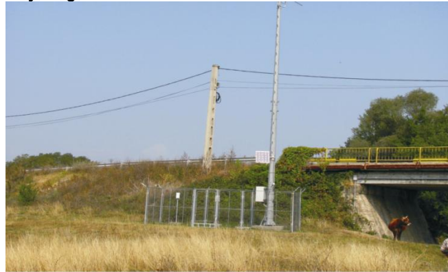
Photo 8. Săcelu automatic station
