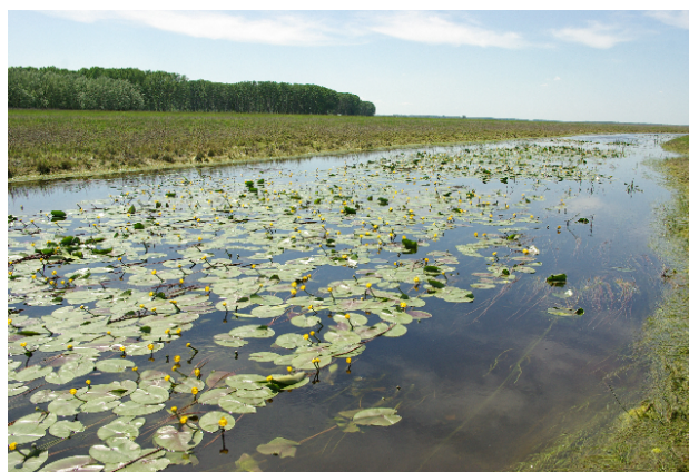
Photo 2. Gerai Pond – a drainage channel, partially clogged.
